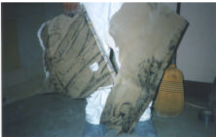
Gypsum board contamination
